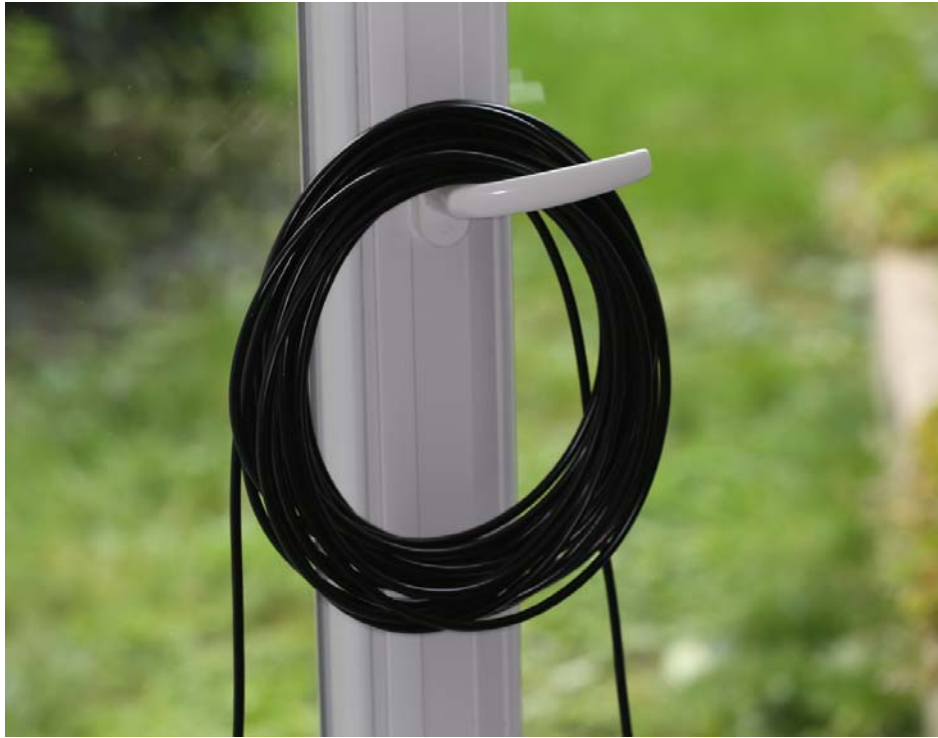
Fig. 13 Avoid to coil the USB and Power cable this way, this increases greatly surge power and may destroy the camera
